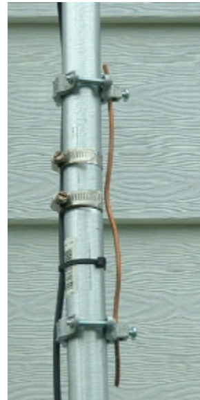
Hose clamps and ground straps at mast joint
